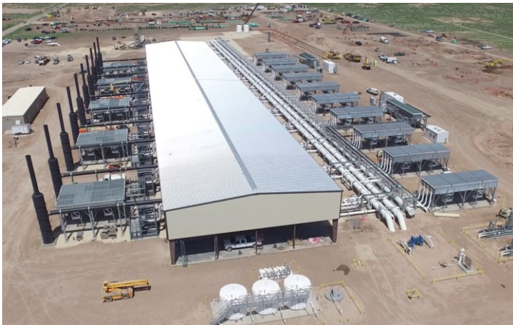
Compressor station operated with ICE
