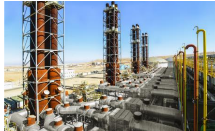
MS engine power plant
